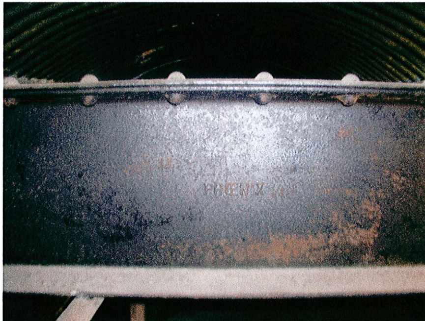
Figure 10 – Turn of the 20th Century Steel Beam Manufactured by Steel Mill ‘PHOENIX’
